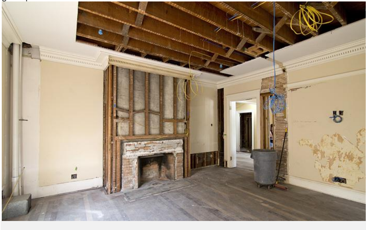
The renovation of a 125-year-old Northwest Portland structure will include the restoration of several ornate fireplaces. (Sam Tenney/DJC)
